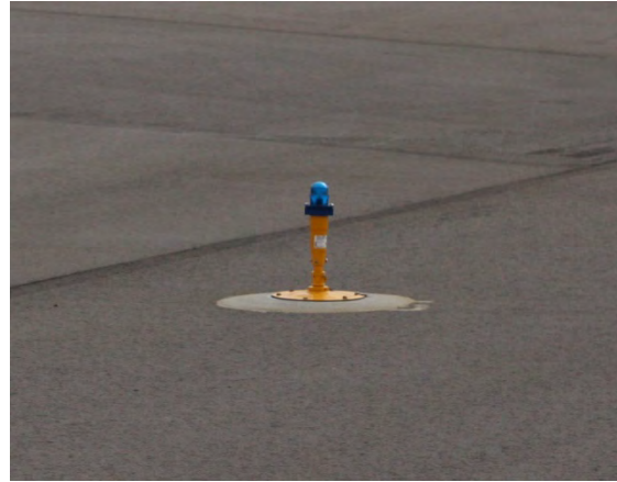
LED Taxiway Edge Light along Taxiway A
