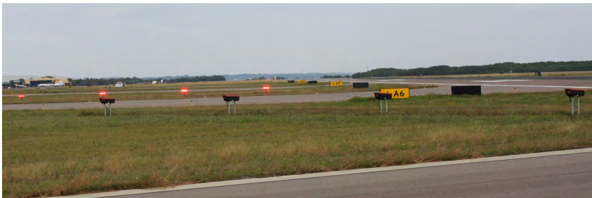
PAPI-4L Systems for Runway 18 (red lights) and Runway 4 (lights not visible)
